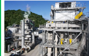
Poultry manure combustion power generation boiler
