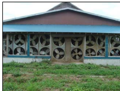
↑牛舎壁面の換気扇
