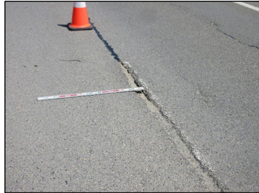
ひび割れ補修跡劣化
